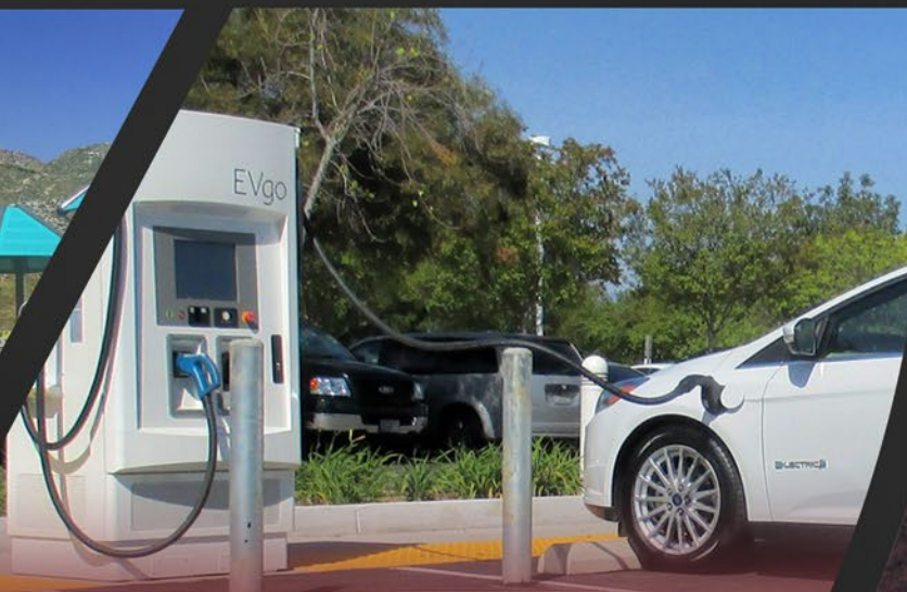
City Hall Electric Vehicle Charging Station
