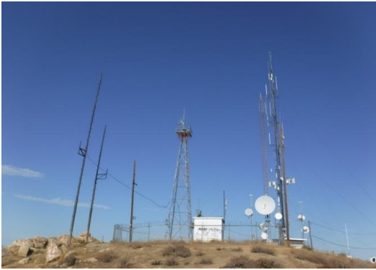
Box Springs Communications Site
