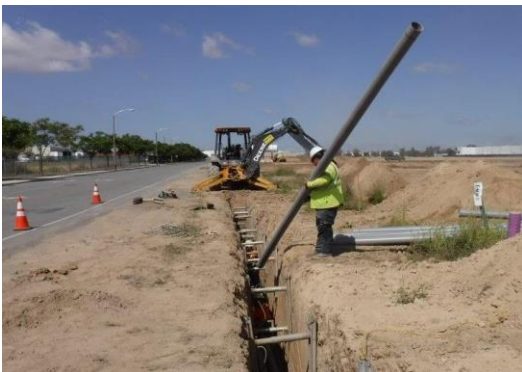
Kitching Substation Feeder Line - Modular 12kV
