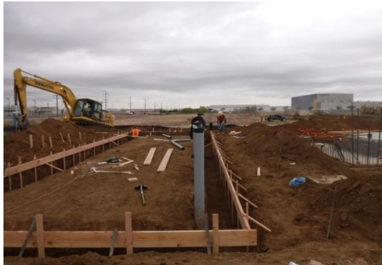
Kitching Substation and SCE Switchyard / Facility Upgrades
