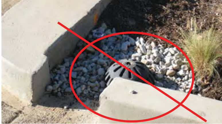
Figure 6: Incorrect Placement of an Overflow Inlet.
